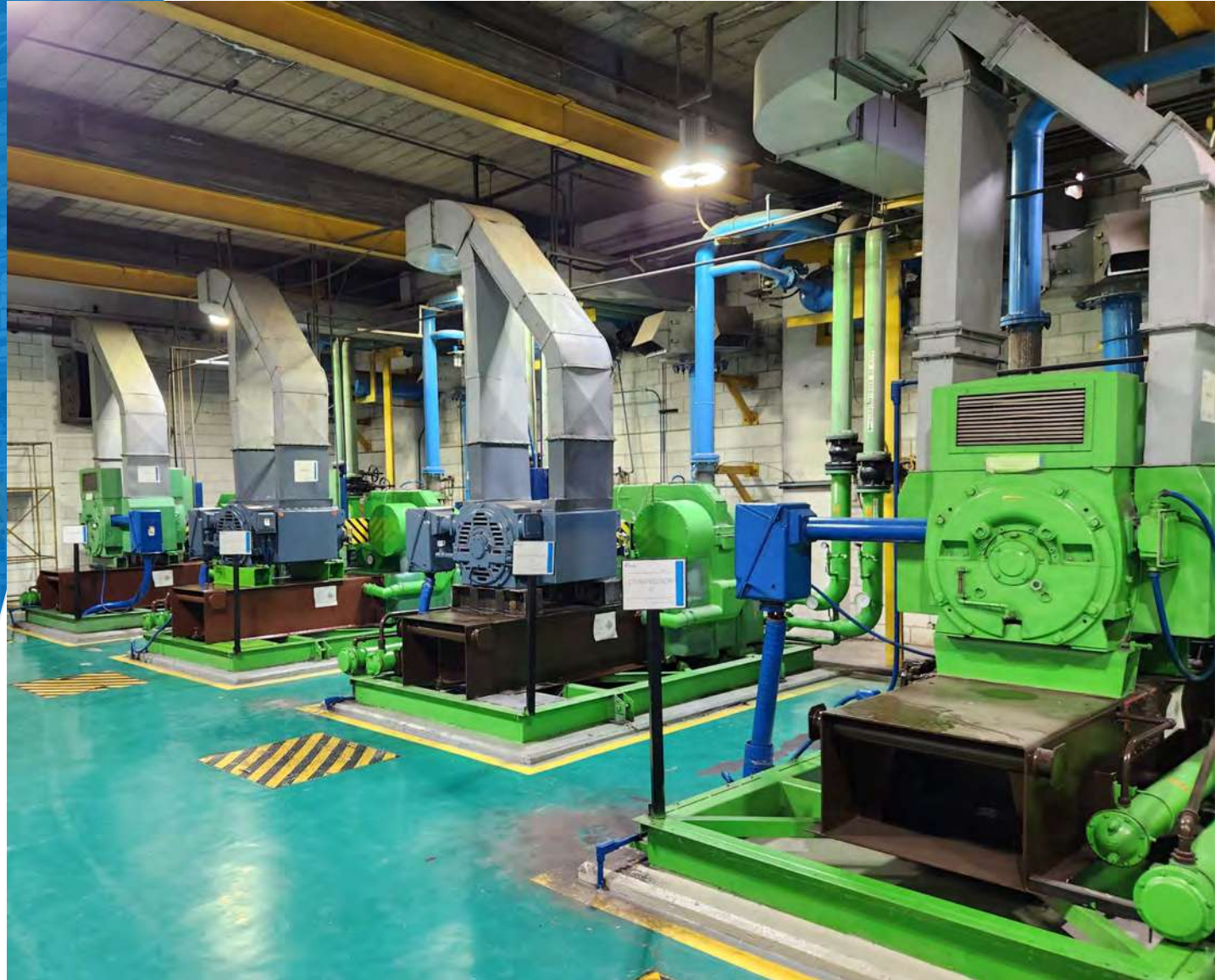
The existing inlet filters on the compressors appears to be undersized
